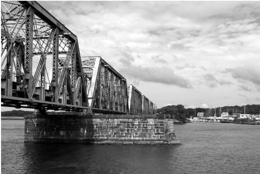
Fixed spans of the Connecticut River Railroad Bridge, Old Lyme - Old Saybrook, camera facing southwest (HPI photograph).
